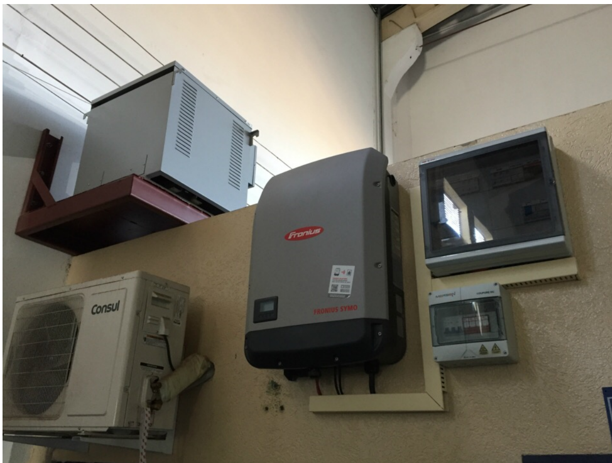
Figura 18 - Inversor Fronius Symo instalado
